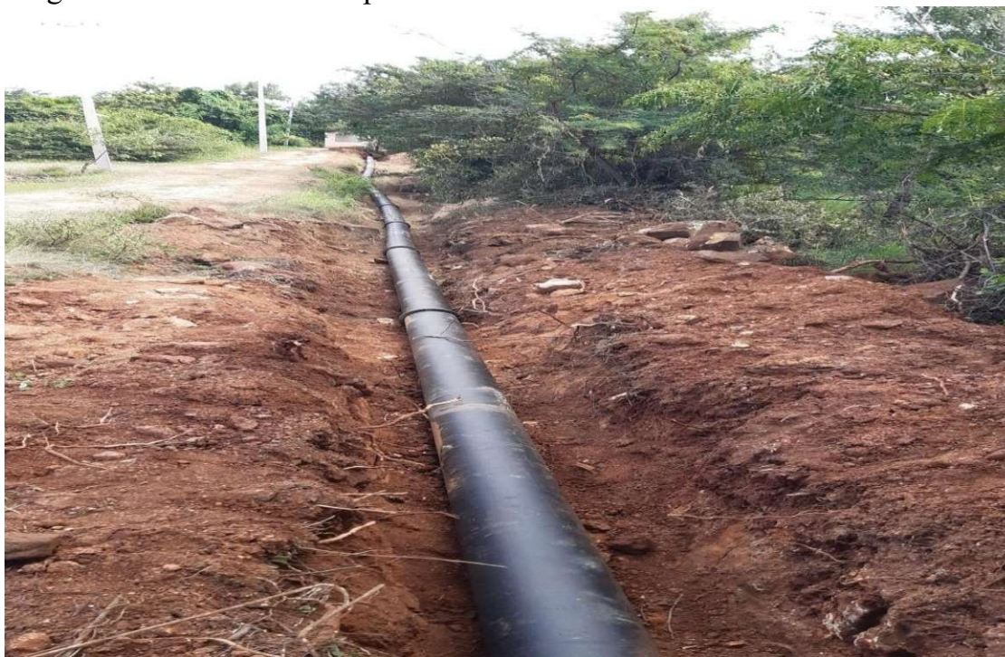
Water pipeline from Tungabhadra River Canal System.
